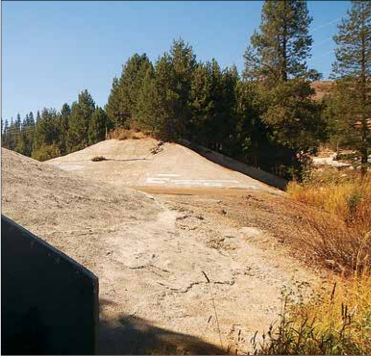
Van Norden Dam is in disrepair and is considered an illegal dam by the State. The Land Trust will lower the spillway height, removing it from the State's jurisdiction, and placing it into a low-hazard classification according to Federal guidelines. Photo by Lori Carpenter.
