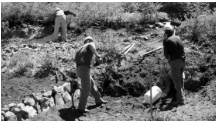
Rock work for the approach to a bridge on the Donner Lake Rim Trail.
