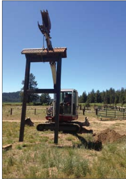
A new trailhead kiosk being installed at the sheep pens in Van Norden Meadow.
