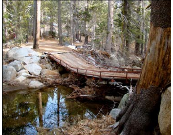
The rickety bridge over Summit Creek will be replaced this summer. Photo by Janet Zipser Zipkin.
